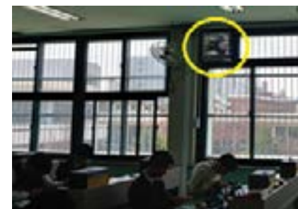
Insufficient ventilation system in a soldering lab
